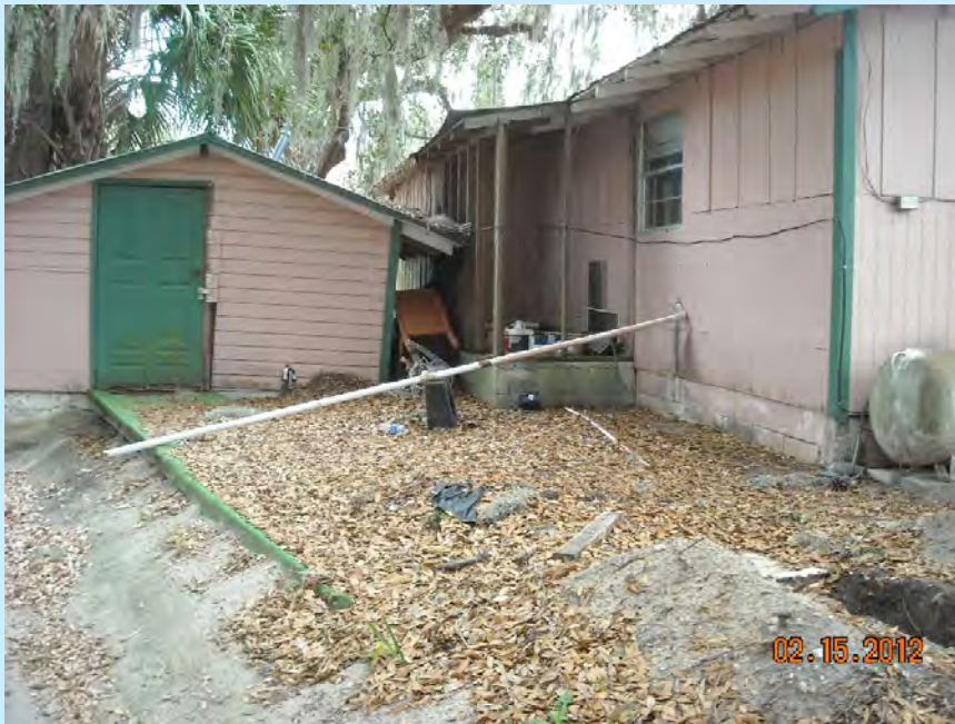
Washing machine discharge
